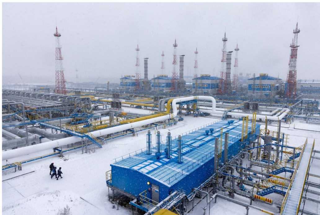
A booster gas compressor station in the Lensk district of the Sakha Republic, Russia. Photographer: Andrey Rudakov/Bloomberg
